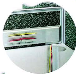
Vertical cabling from floor
