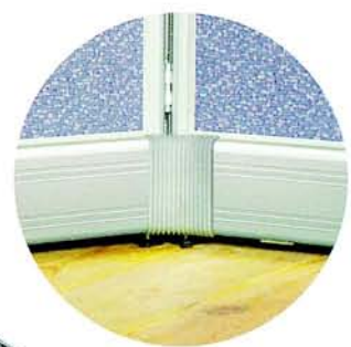
Continuous cabling between screens
