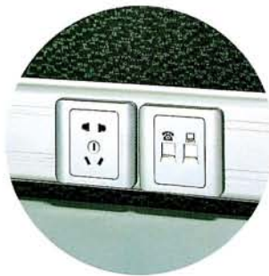
Power sockets installed on cable channels
