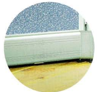
Cabling in raceway
